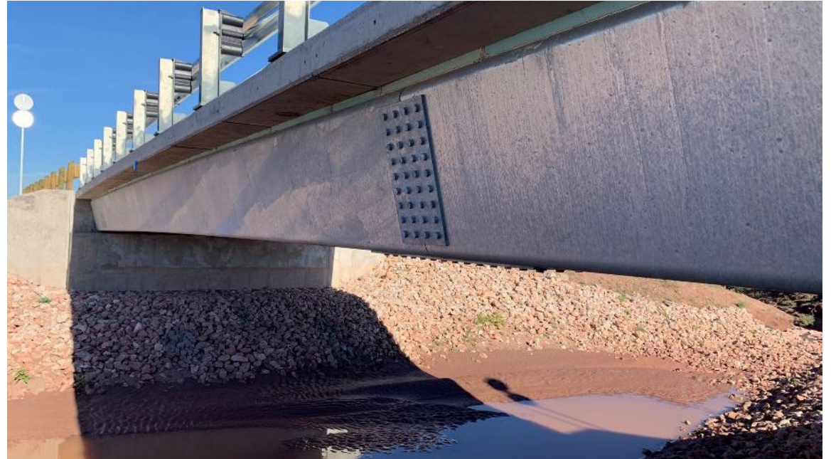
USACE Fort Wingate Bridge Replacement Gallup, NM | 2022 52 tons – Press-brake-formed steel tub girder: 8 beams weighing 12,600 lbs. each
